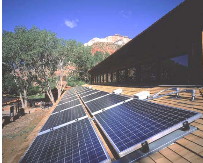
Figure 4-11 PV panels installed on the roof at the Visitor Center
