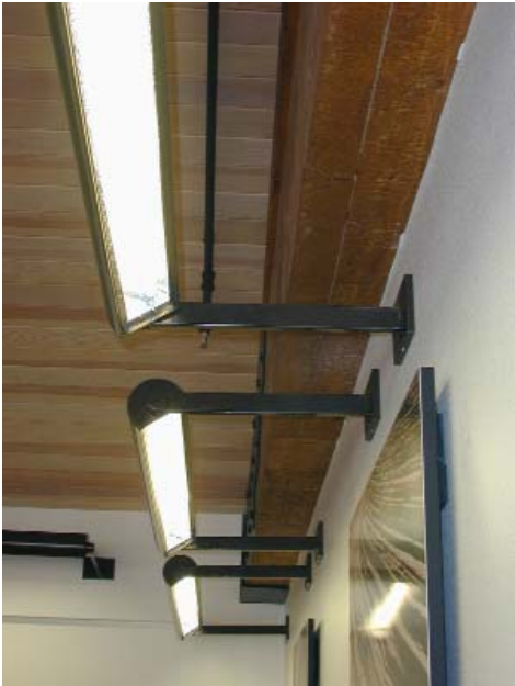
Figure 4-6 Display lighting using 4-ft T-8 Lamps
