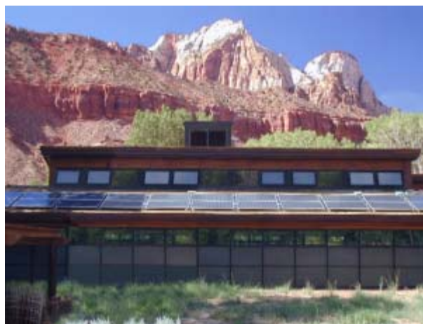
Figure 6-15 Photo of shaded PV panels (left side of photo)
