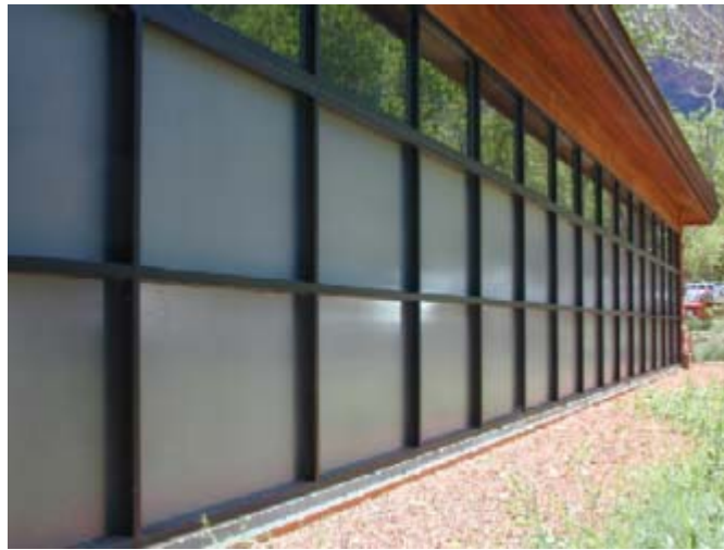
Figure 4-14 Photograph of Trombe wall showing patterned glass over the Trombe wall, row of daylighting glass, and overhang to shade wall during the summer
